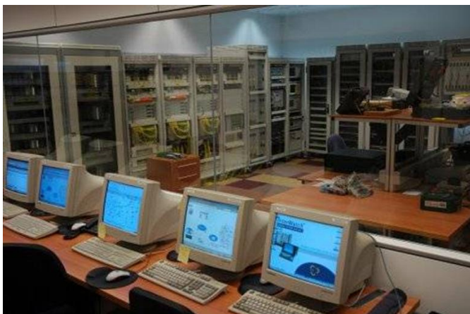
Fig. 3. The ADRENALINE+ testbed
