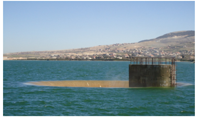
Fig. 5. Flood relief through the spillway of the Qaraoun dam
